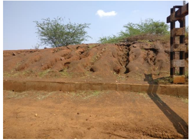
Pic. 12 – Raincuts resulting in silting up of bridge
