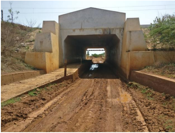
Pic. 11 – Silted up bridge
