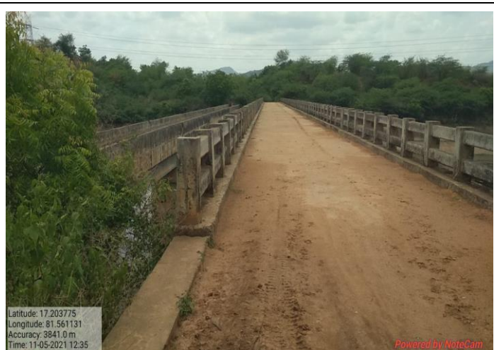
Photo showing view of the Single Lane Road Bridge at km 8.135 of RMC from left bank of canal
