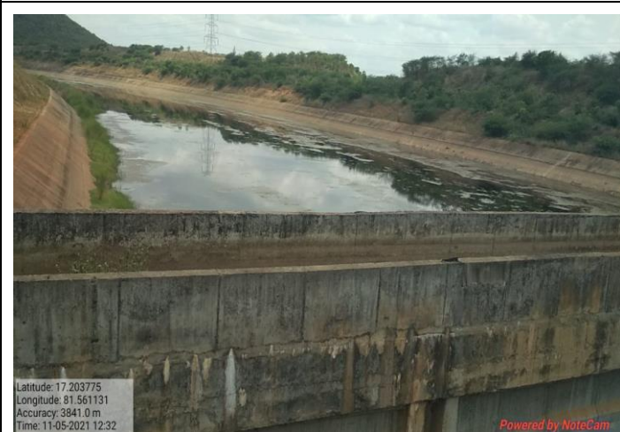
Photo showing view of the Super Passage at km 8.135 of RMC from upstream of canal
