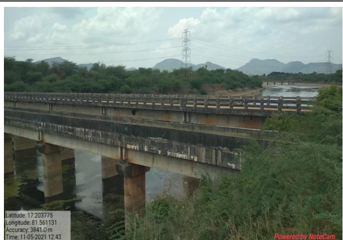
Photo showing view of the Super Passage cum Single Lane Road Bridge at km 8.135 of RMC from Downstream of canal
