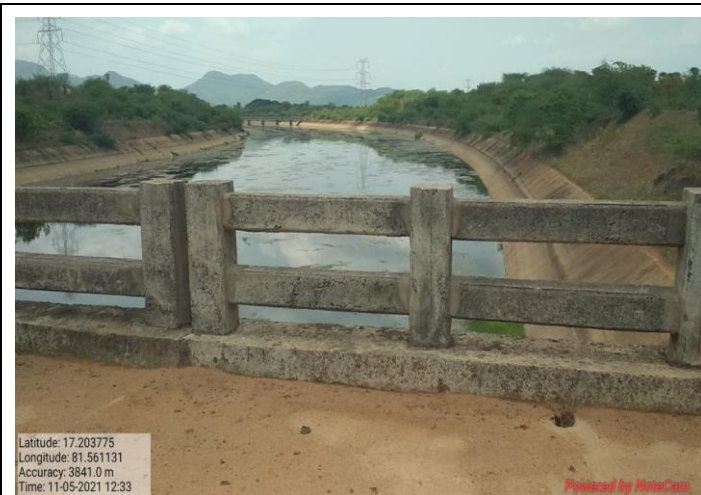
Photo showing view of canal from the top of the Single Lane Road Bridge at km 8.135 of RMC
